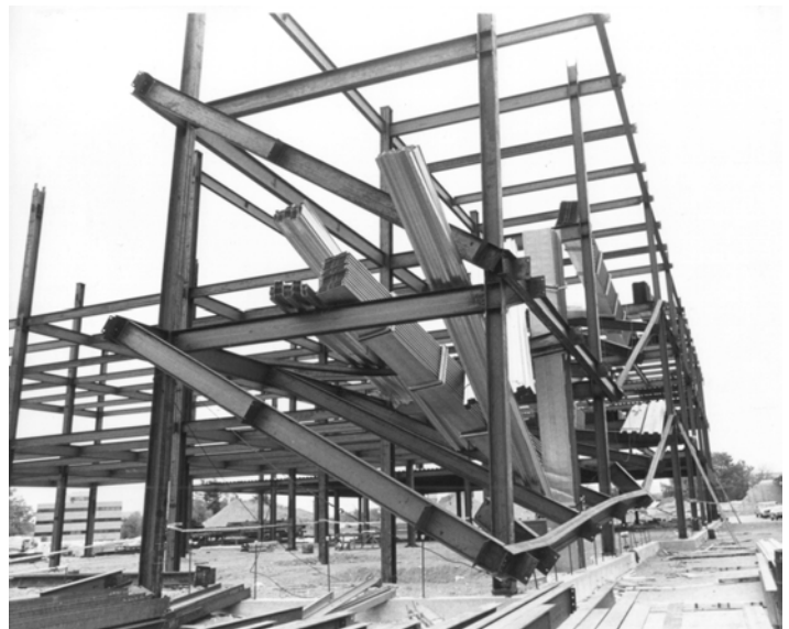
Figure 2. View of collapse at northwest corner of the building, taken prior to the removal of debris.
