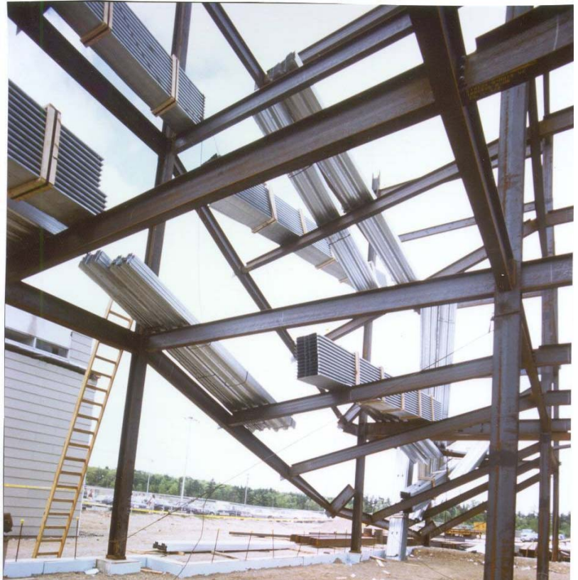
Figure 7. View of collapse looking northwest.
