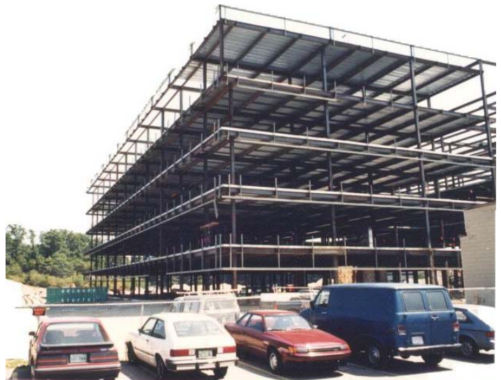
Figure 1. View of the northwest corner of the building, showing the area where the steel framing collapsed during erection.
