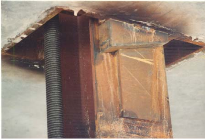
Figure 2 Detail at bottom of steel lifting collar. Slab temporarily parked. One of two lifting rods is shown on left; other rod is hidden on other side of column. Left and right sides of lifting collar extend beyond opening at bottom of slab, but extensions are hidden by cement paste.
