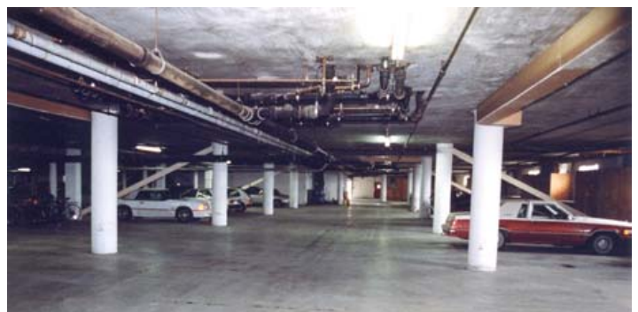
Figure 11 Typical flat bar diagonals of braced frames in condominium buildings; diagonals shown are in basement story of Building B. Columns are steel, but are encased in concrete in the basement garage.
