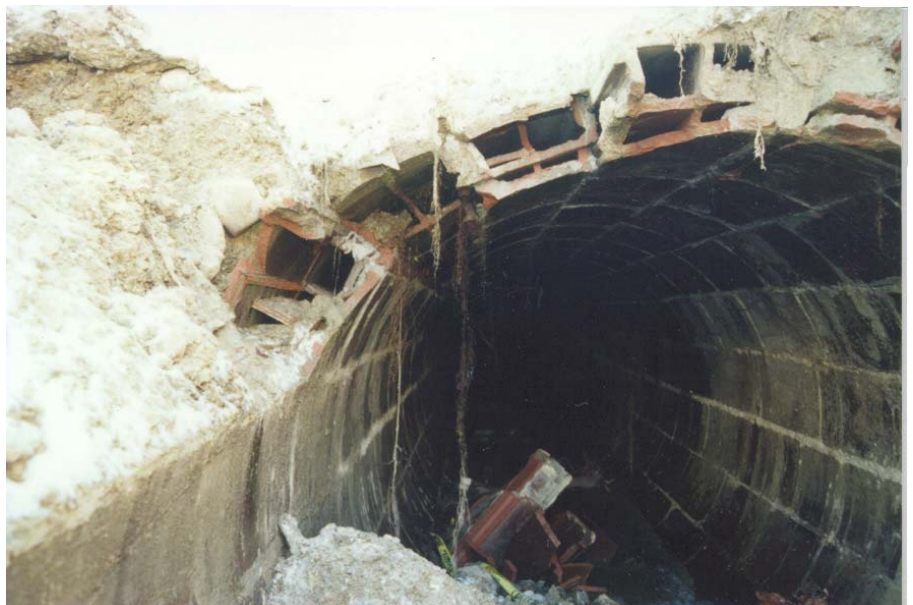
Figure 4. West end of collapsed storm sewer, showing details of the clay tile construction.
