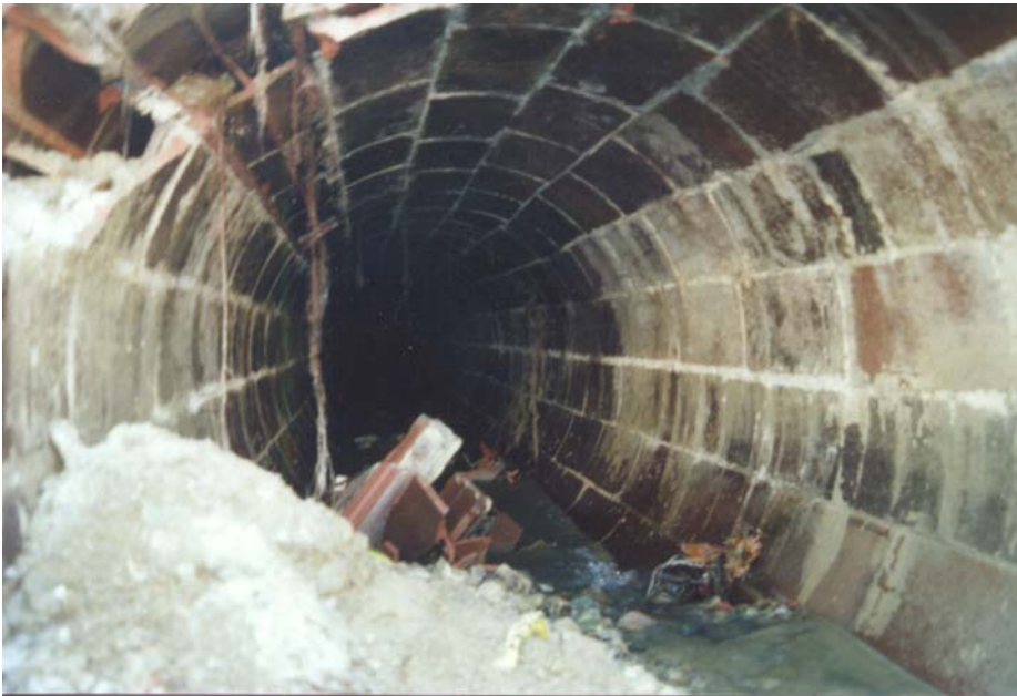
Figure 1. Trunk storm sewer west of the collapse, showing structural clay tile construction. The sewer is 5'-6" in diameter and there are 18 tiles around the circumference
