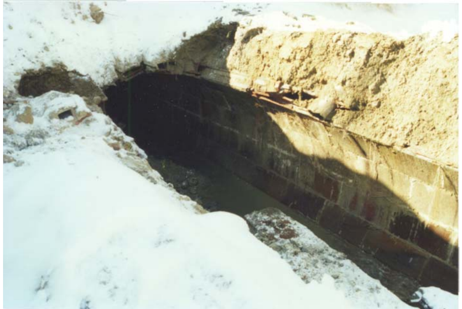
Figure 3. Collapsed storm sewer at the west end of the collapse, looking northwest.
