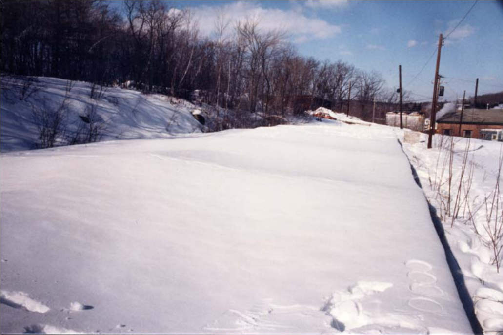
Figure 4. View of the collapsed roof, the day after the collapse. The collapse was arrested by a thick layer of ice at the top of the pond.
