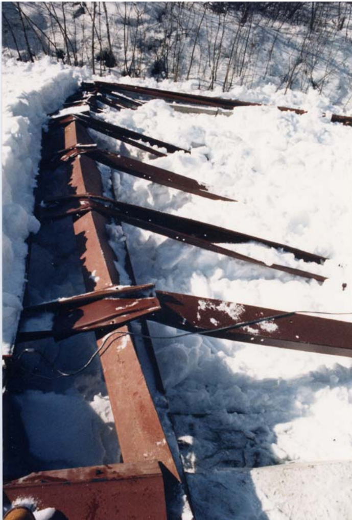
Figure 1. View of collapse of roof over chemical settling pond, showing a typical condition of the framing. All the light gage steel purlins across the entire width of the roof have rolled over away from the viewer.
