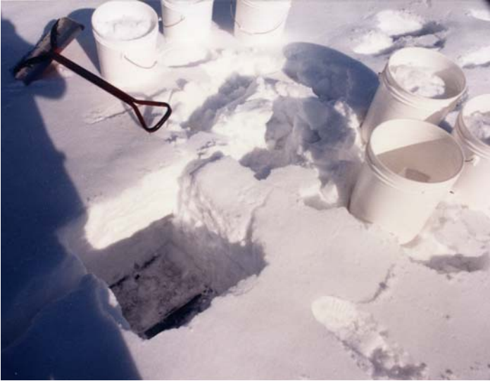
Figure 5. Test hole in the snow on the roof, to determine the density of the snow.
