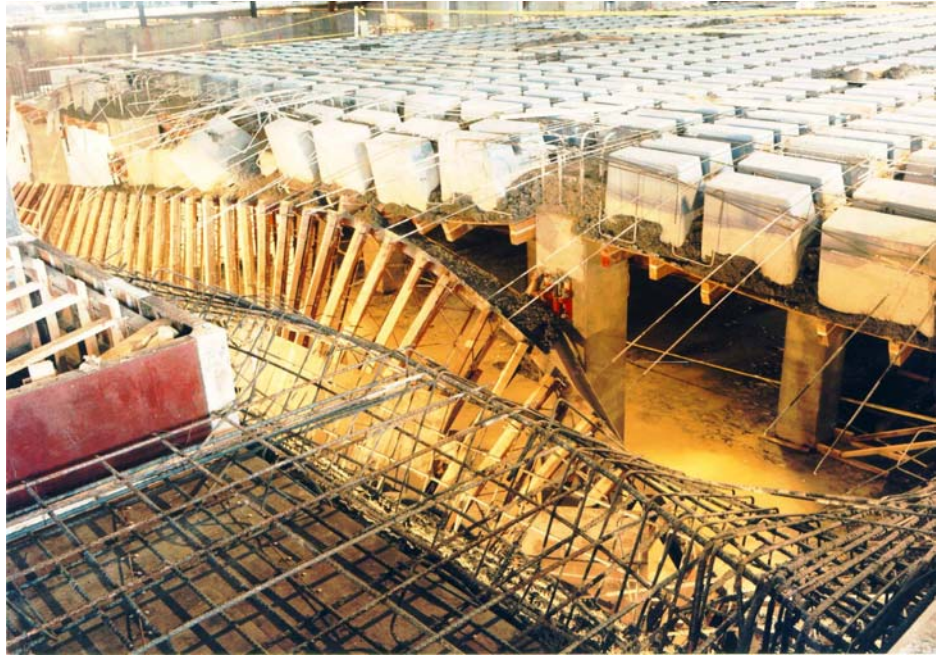
Figure 9. View of collapse, looking eastward.
