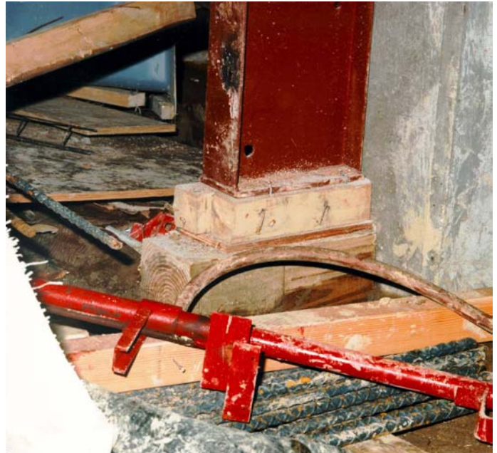
Figure 7. Wood blocking supporting base plate of temporary steel column on Line 5; believed to be at the most northerly end of the formwork that collapsed. (The column shown did not collapse).
